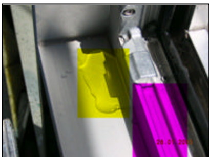
Fig 9 An example of a high quality european window with major leaking problems due to poor shop and field workmanship and a lack of comprehension from the supplier.
